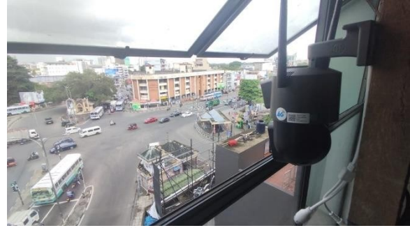
Fig. 3. Camera installed at the junction
